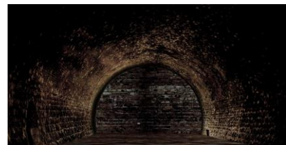
V25 Old Joe (sewer pipe)
